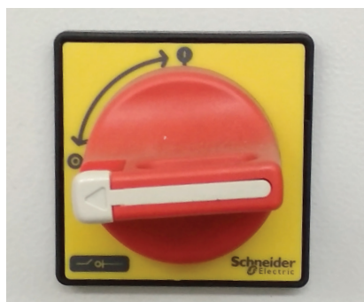
Figure 40 Main electric switch
