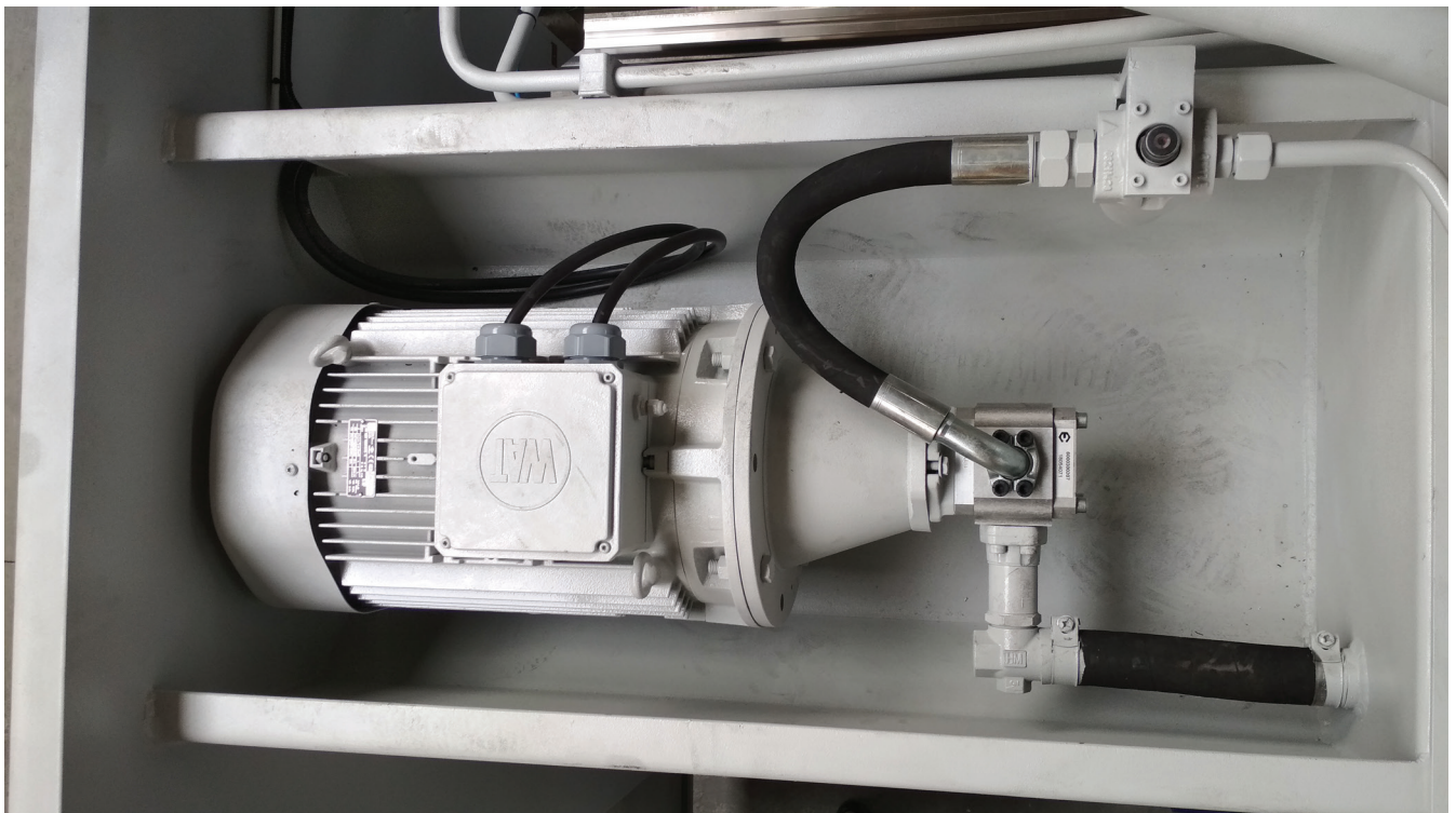
Figure 65 Main motor, pump and filter
